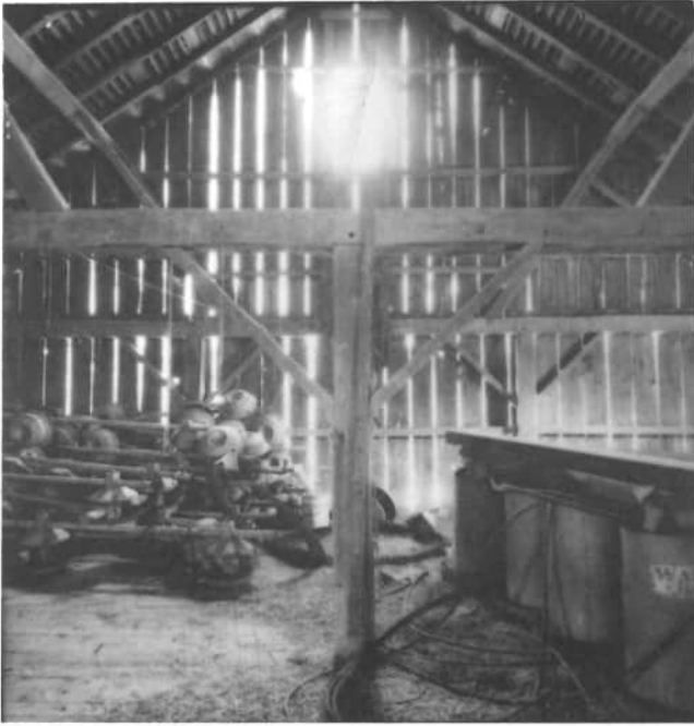
An interior view of Tom Olding's barn, shows the cross beam, with inclined purlin posts beneath the rafters. The sunlight accents the vertical siding. (Andrew Pax photograph)
