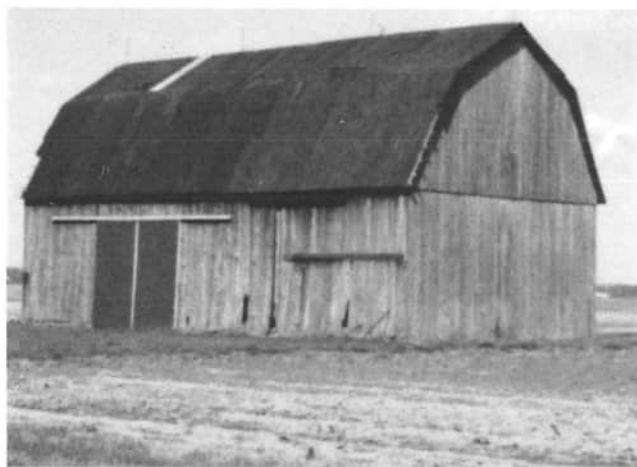
Fred and Rose Meyers built this barn in 1906; the barn stands on State Route 49, and is owned by Harold Muhlenkamp, 8058 State Route 49, Celina. In the past the barn was used for livestock, hay, and grain; today, the barn is used for machinery.
