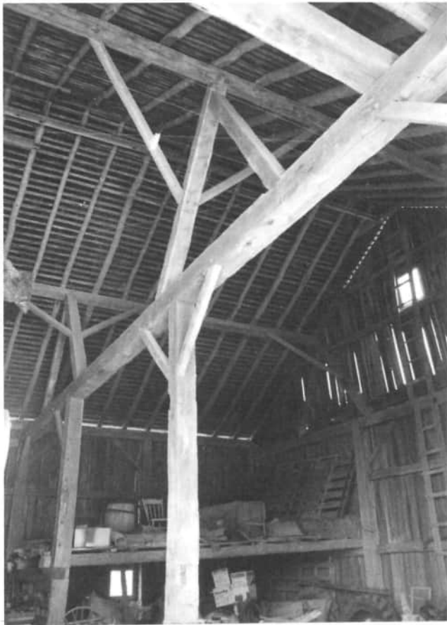
Another view of the support frame of Eugene Behm's barn, 89 Strable Road, Rockford. Note tree limbs supporting the rafters.
