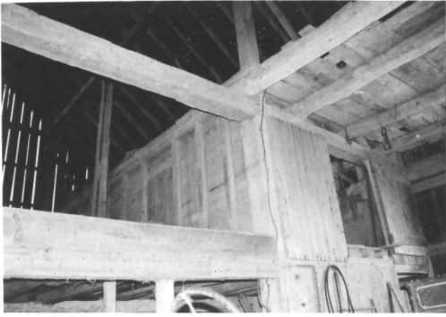
This interior view of John Homan's barn, 97 Elm Road, not only shows the big cross beams, but also the grain bin.
