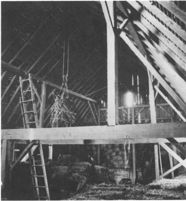
An interior view of the haymow, shows the huge cross support beams, which support the roof. The ladder is resting while the mow is standing almost empty. The old hay rack is still attached to the pulley, which hangs from the ridge pole of the roof. The gambrel roof gives more space in the mow, at the barn of Lou Ann Timmerman, 3157 Township Line Road, St. Henry. (Andrew Pax photograph)
