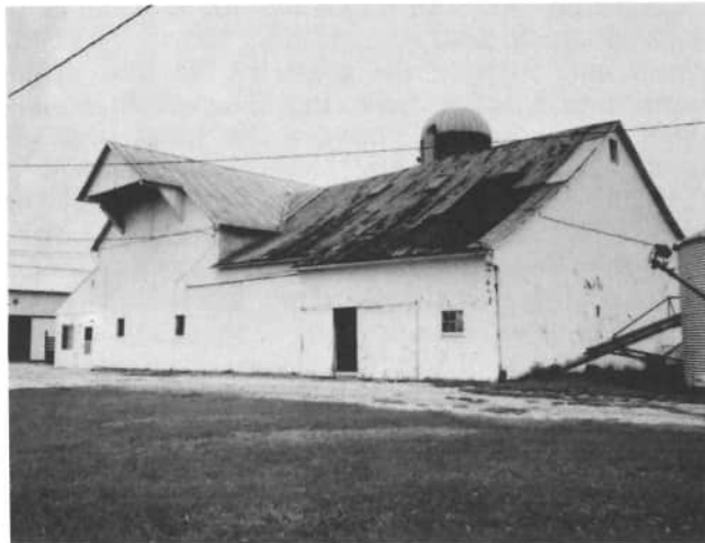
John Guggenbiller's barn, 1111 Township Line Road, Saint Henry, was built in 1900. The barn was used for milking cows in the stable, grain storage, straw and hay storage, and farrowing sows. Today, the barn is used as a holding pen for cows, feeding baby calves, and for straw storage.
