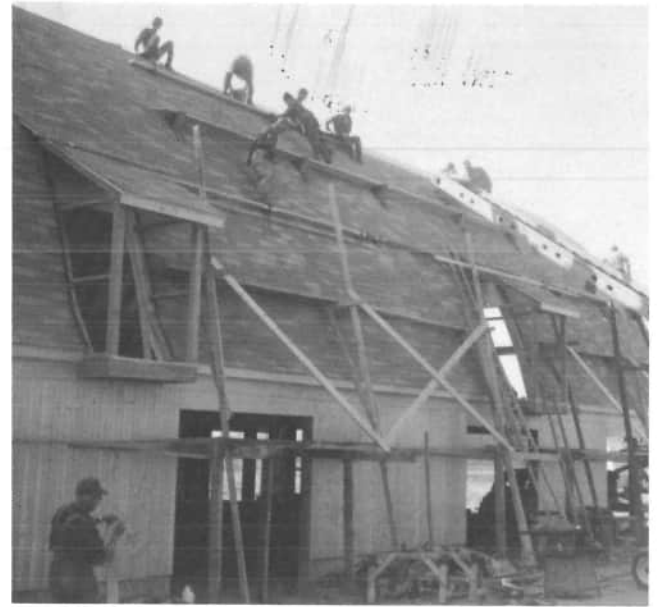
The roof on Ivo Siegrist's barn is receiving its finishing touches; many hands made the work go quicker. The two shed roofed dormers are beginning to take shape on this photograph.
