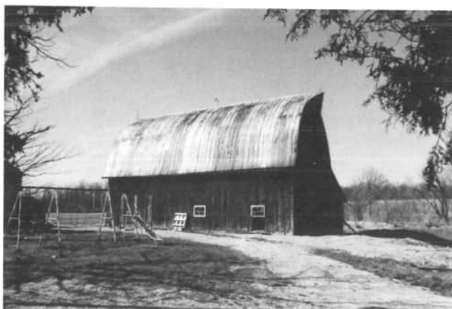
John Meinerding, 8809 State Route 197, Celina, owns this red barn. The weathered metal roof has the hay hood extended over the end wall. The swing set in front of the barn reminds us that children are about, which reminds those of us who had the childhood pleasures of playing in the haymows and running the rafters.
