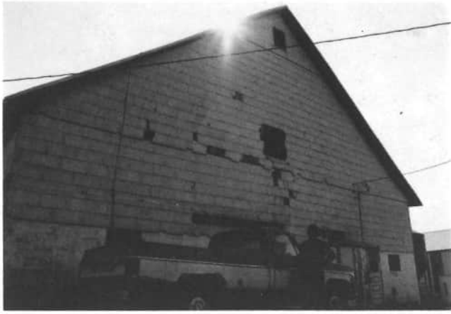
Andrew Schlarman, 1919 Clune-Stucke Road, stands outside his barn, at 1818 Clune-Stucke Road, where his son Larry lives. This barn has served the purposes of agriculture for the five generations of farmers that have used it; namely, John, who built the barn; Henry; Lawrence; Andrew; and now his son Larry Schlarman.
