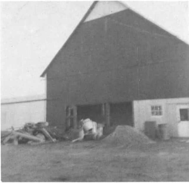
This June 1966 photograph shows work in progress at the Luke Broering barn.
