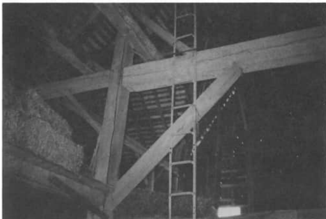
An interior view of Virgil Franck's barn shows the huge post and braced beam, making up one of the bents which support the roof. Note the wooden pins in the post.
