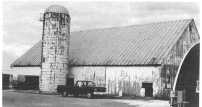
This barn is 96 feet long, 50 feet wide, and 38 feet high, and is now setting on the Steve and Nancy Broering farm. The barn will soon be moved to the Dale and Bonnie Dippold farm. The plans for the barn are to raise steers and hogs in it; they will also use the barn for storage of machinery, hay, straw, and other needed storage.
