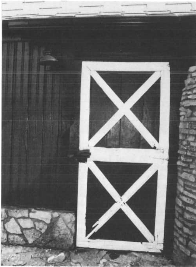
A view of a side entry door at Carl Jackson's barn shows the X bracing on the upper and lower sections of the door.
