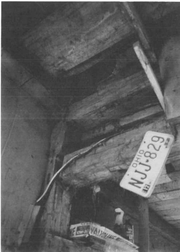
This interior view of the Louis Zizelman barn shows the corner notching, as well as the wooden pegs which pinned the posts and beams. The outside of this barn makes it appear to be just another small building; but inside, the framing is a historical treasure.
