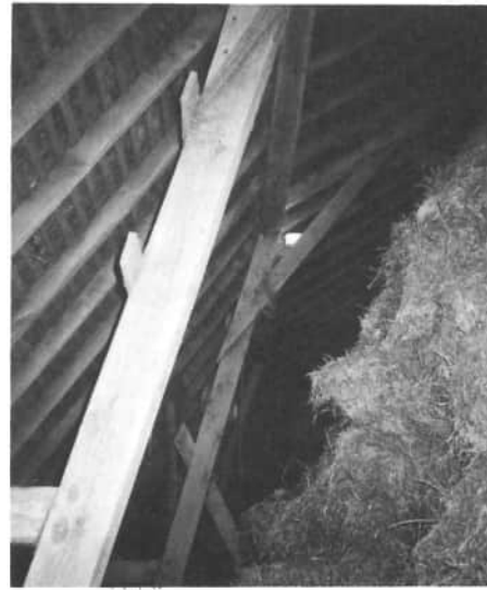
An interior view of the Huwer barn shows the supporting posts of the rafters of the gambrel roof, and how there is more room in the mow.
