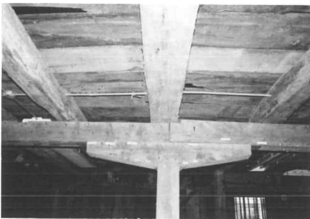
This interior view of Carl Jackson's barn shows the cross beam beneath the mow, being supported by an additional beam above the vertical post.
