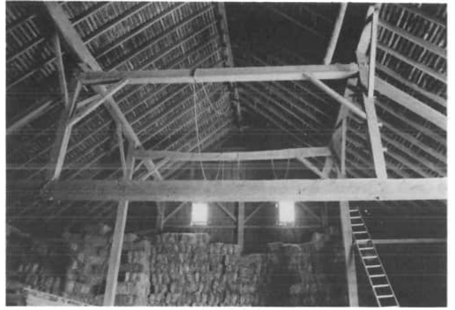
This interior view of John Fleck's barn shows the major cross beam has no support beneath it in the center, but it supports the posts which support the purlin. Note the vertical post is cut to extend through the cross beam, and pinned with wooden pins.
