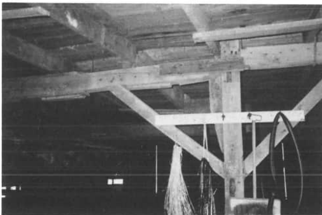
Another interview shot shows the support structure, with a twentieth century snow shovel asleep between seasons.
