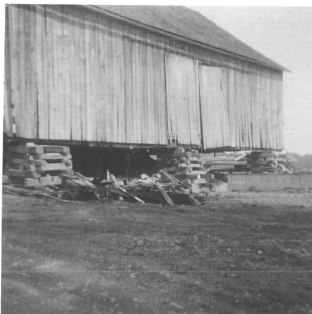
The moving of the barn was begun on June 1, and completed June 7; they worked on it about four days.
