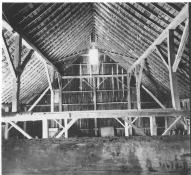
An interior view of the Stachler barn at 1333 Sharpsburg Road, shows the height of the posts supporting the purlin plate beneath the rafters of the barn. The sunlight outlines the vertical siding on the end of the barn. This symmetrical photograph was accomplished by professional photographer Andrew Pax.
