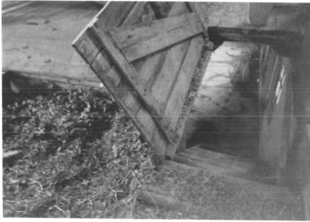
This interior view of the John Tobens' barn, shows the opened door of the floor, leading to the basement or ground floor of this grundscheier barn. The steps are wood. Next to this basement door, is the wood threshing floor of the main floor of the barn. This was a grand barn in its day.
