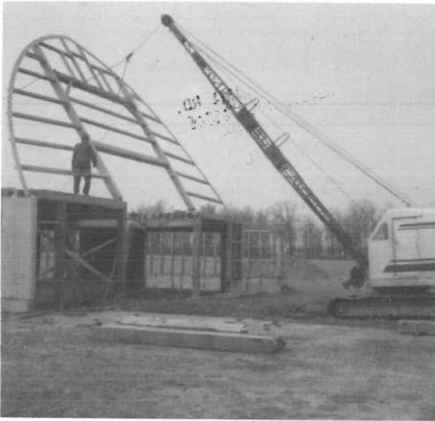
Ray Staugler and the neighbors held a barn raising at Ivo Siegrist's place in 1971. In the 1970's a crane is used to raise the end wall into place. (In the 1870's, this power would have been provided by man and horses.)
