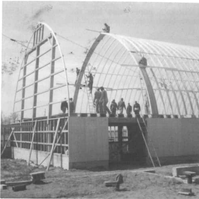
Ivo Siegrist had his barn built on the same site as the old barn, but he put in a new foundation, and, instead of a gable roof, he put on a round, or gothic roof, in order to have more room in the mow. Family and neighbors are helping, but who volunteered to sit on the ridge pole to work?
