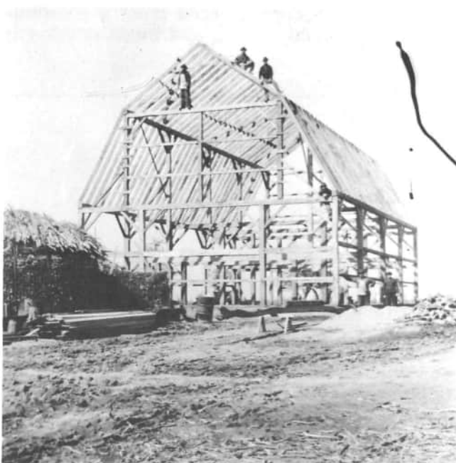
This is a view of the framing of the Hemmelgarn barn, 1551 Cranberry Road, St. Henry. On the end wall, note the vertical posts on the bottom floor supporting the cross beam, which supports more vertical posts which support the purlin plate (the beam which runs the length of the barn supporting the rafters). Note how the carpenters nailed cross boards to the vertical posts, for easier climbing to the rafters of the gambrel roof. No fear of heights was needed for the barn builders. Frank Hemmelgarn's son David Hemmelgarn, 5395 Fort Recovery Minster Road, owns the place today.
