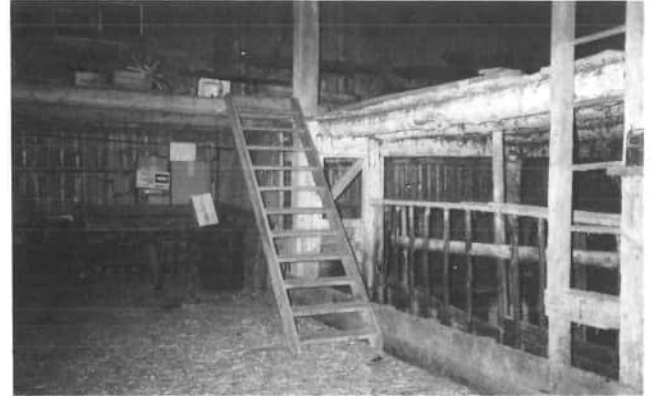
An interior view of the east half-mow and south haymow, of Jim Homan's barn.
