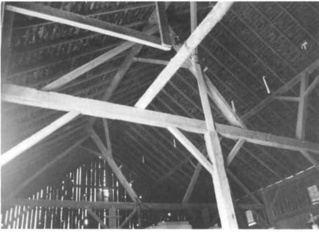
Another view of Edson Pierstorff's barn not only shows the inclined support posts for the purlin, but also shows the stepping boards on the posts to climb higher in the mow.
