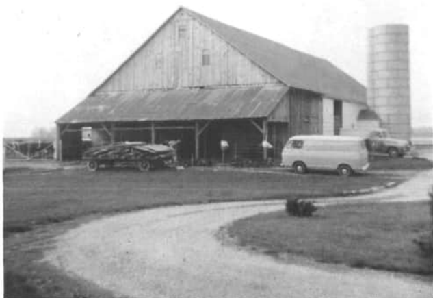
This view of Donald Unrast's barn shows the Stachlers, of Ray Stachler Construction, working on the barn.
