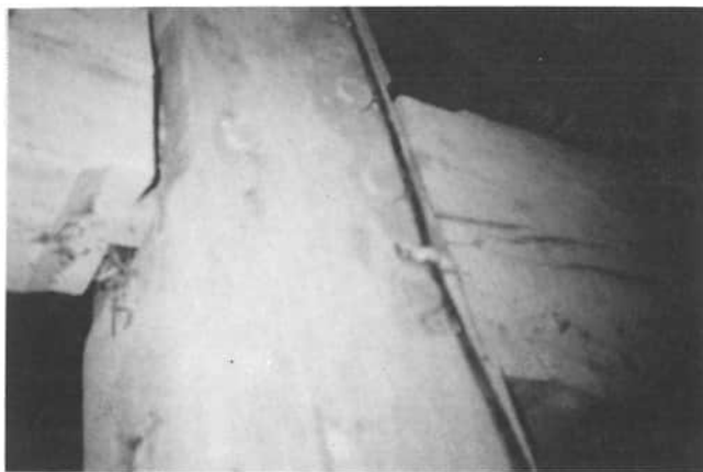
A close-up of the post, whereby the mortise was cut to receive the tenon of the beam, and was securely fastened by wooden pins, in the Franck barn.
