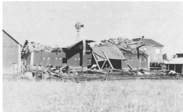
Another view of Lloyd Schwieterman's place after the July 19, 1952 storm. Note the number of stable doors across the back of this barn. Note the damage to the blades of the windmill, or otherwise called the windpump. Note the other buildings.
