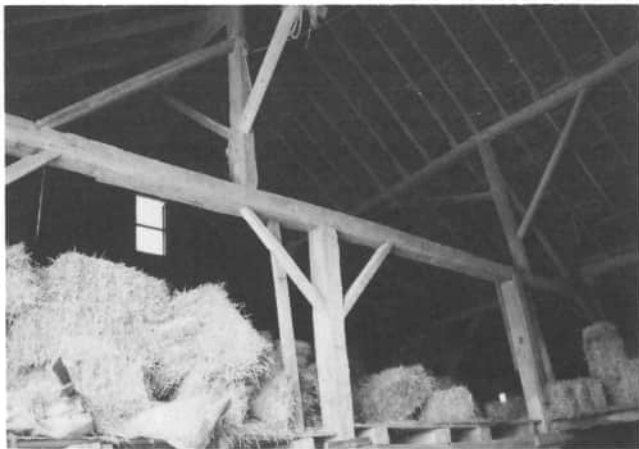
This interior view of Fred Dues barn on 3691 Township Line Road, shows the hugh cross beam, and the vertical posts which support the roof.
