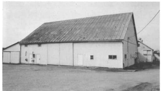
This farm and barn have been owned by nine different owners, but they have been basically used for general farming. In 1947, a tornado came through this area and moved the barn partly off of its flagstone foundation and pushed the top eighteen inches out of square. With jacks, and other miscellaneous equipment, it was almost straightened out. It is still about four inches out of square. The barn was built in the late 1800's by Frank Kunk. Today the barn is used for swine production. The barn belongs to Edward and Robert Pohlman, 1194 State Route 716, Maria Stein.
