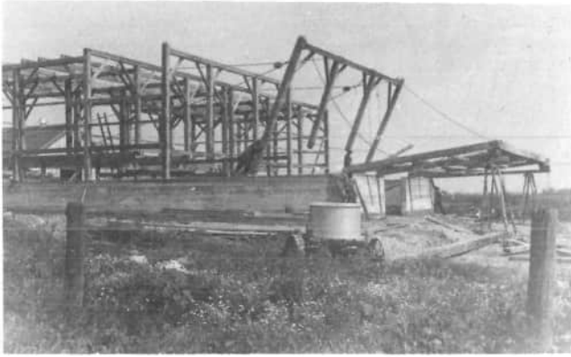
This old photograph of Patrick Schmitmeyer's barn, 4321 Guadalupe Road, shows the last span of the east wing being erected on a Saturday morning in June 1941.
