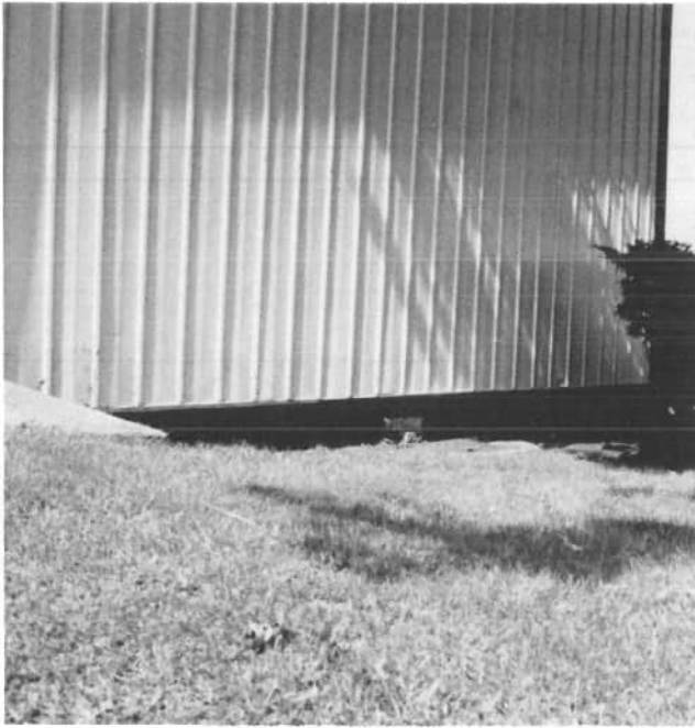
This is a close up view of the stone foundation of Wayne Shively's barn, 8675 State Route 118, Celina.
