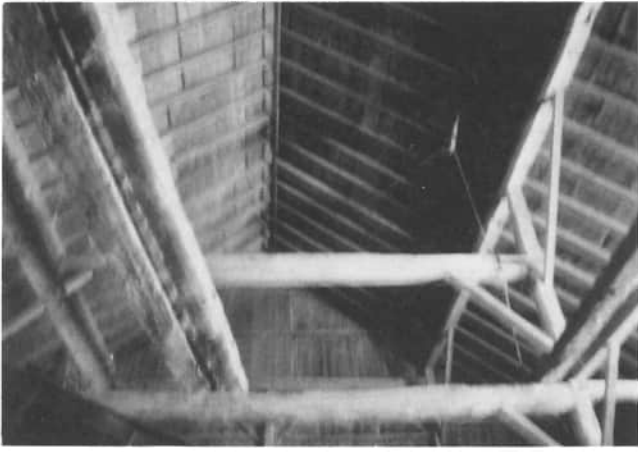
This interior view of Louis Bertke's barn shows the framing of this big barn.
