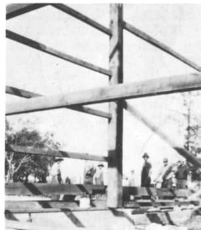
This is a late August 1932 view of the Huwer barn, as the tenons of the beams are being fit into the mortises of the posts of the main frame bents.
