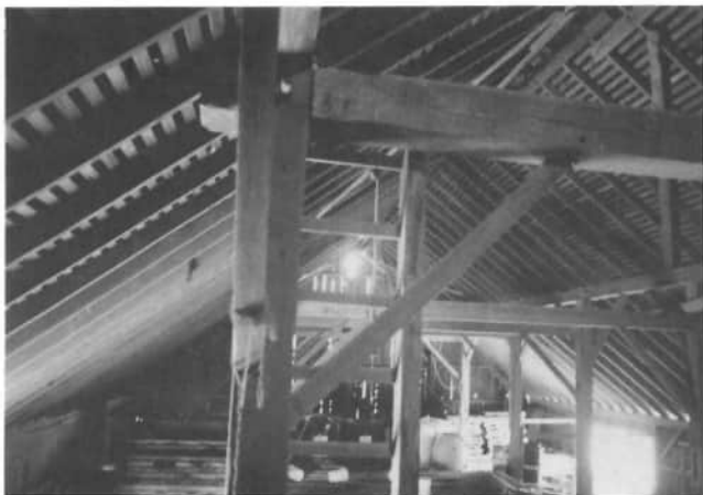
A close-up view of the tenon extending through the mortise, being pinned with the wooden pin. The vertical post supports the purlin, in the Stucke barn, 501-Clune-Stucke Road. The cross can be seen in the end wall.
