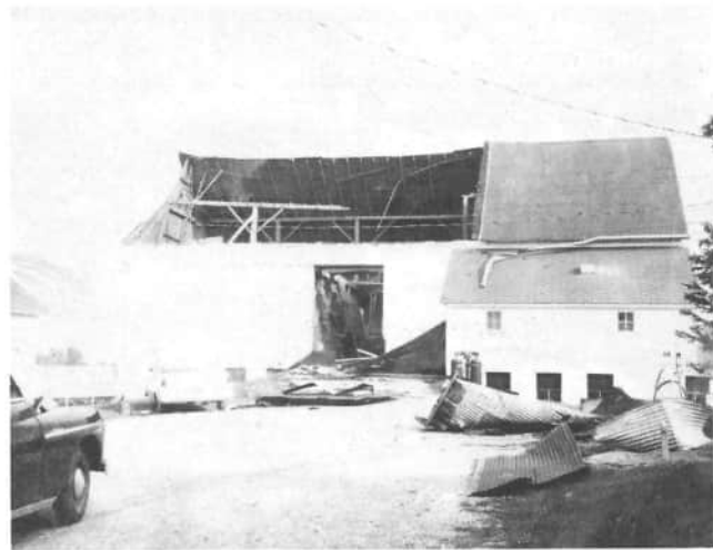
Ivo Goettemoeller's barn was hit by a tornado in 1960. The roof was twisted off and strewn about the barnyard. The top part was rebuilt.
