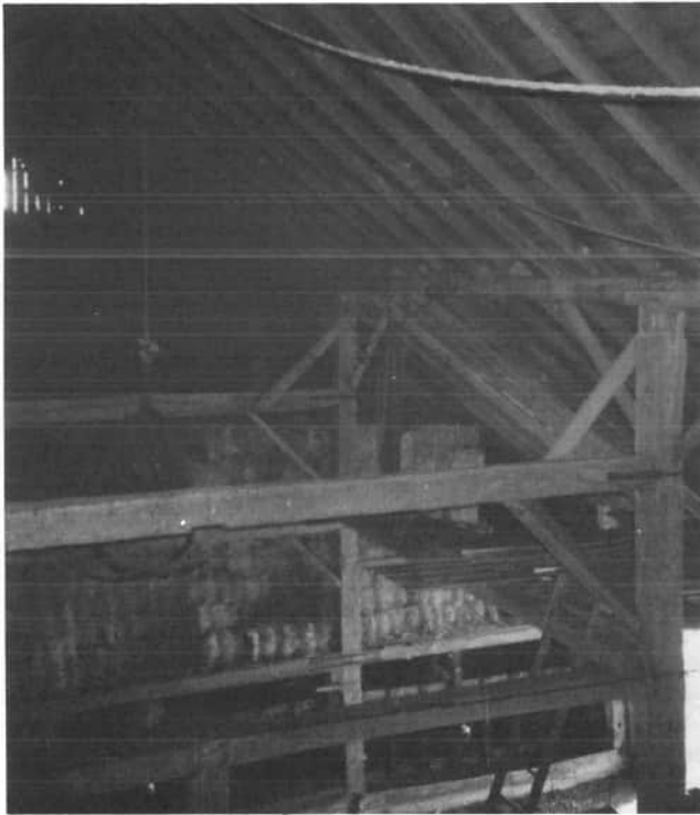
This interior view of Carl Koesters' barn, 6440 Fort Recovery-Minster Road, shows the framing of the barn, with the vertical posts, and the lower cross beam extending from wall to wall, and the upper cross beams extending only to the vertical posts supporting purlin plate beneath the rafters.
