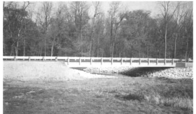
New Prestressed Concrete Bridge on Neptune-Mendon Road. One of 91 built in the past 9 years.
