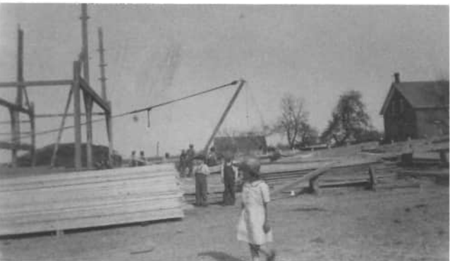
Mrs. Henry Pohlman had this barn built the summer of 1940. Bill Wellman, Sr., Father of Bill & Bernard Wellman, built this barn. The men are hooking up a bent, getting it ready to raise.
