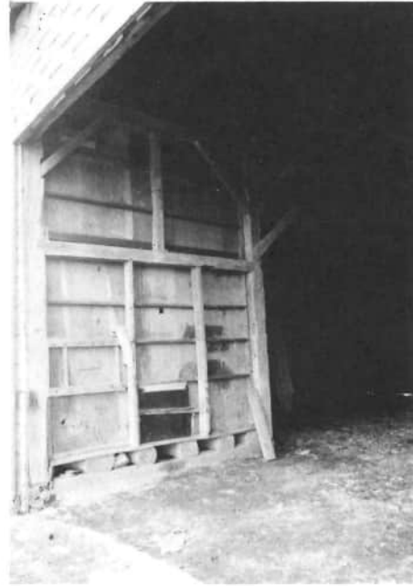
This interior view of Olan Stoner's barn on Hayes Road, gives a view of the grain bin, which was used for shelled corn or wheat or beans. Note the base whereby logs are used for the floor support. The posts are hand hewn and wooden pinned.
