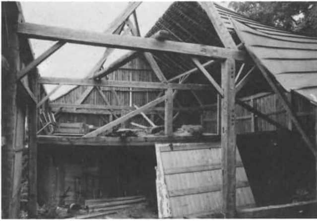
This photograph of the Wenker barn shows its frame, as being one of the few barns, with incline support posts for the purlin, beneath the roof.
