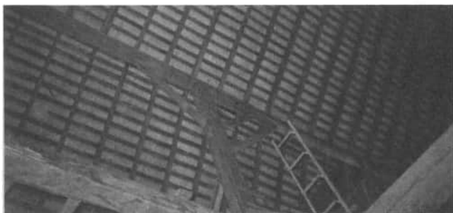
An interior view of Virgil Franck's barn shows the post supporting the purlin, which supports the rafters, of the gambrel roof.
