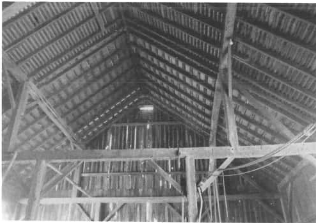
An interior view of Glen and Dorothy Miller's barn, 9926 State Route 118, shows the framing of the barn. The notches on the main cross beam indicate the beam was hand hewn. The vertical posts above the cross beam, support the purlin plate which runs the length of the barn and supports the rafters.
