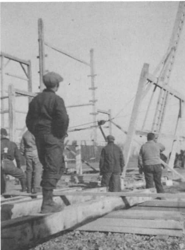
The main bents of the barn are being raised into place by Greg Prenger, Frank Prenger, and their neighbors.
