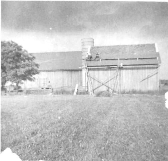
This is an old photograph of the Luke Broering barn. The barn was reroofed three times. The original roof had wooden shingles; then, it was reroofed with asphalt shingles. Then, they stripped it and put metal on the roof.
