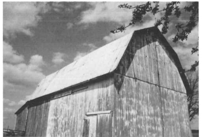
Chris Weitz's barn, 2431 Frahm Pike, Celina, was built in the early 1900's. The weathered barn has gained a silver patina. An addition was made to the left end. A protection of vertical boards was built over the track above the double doors. In the past, the barn has been used for horse and cow stables, farm machinery storage, and a hay loft. Today, the barn is used for storage.
