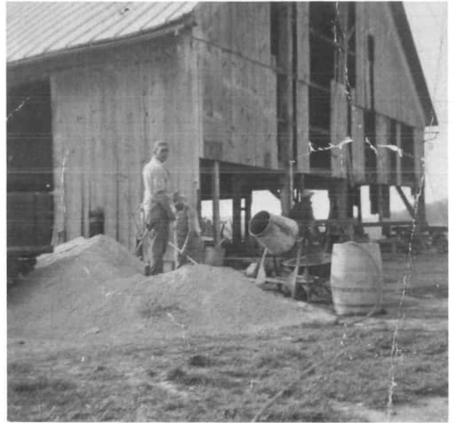
Another view in May 1955 shows the Amish crew helping to put the barn on a cement foundation and to reside the barn, at the Menchhofer farm at 1151 St. Anthony Road.
